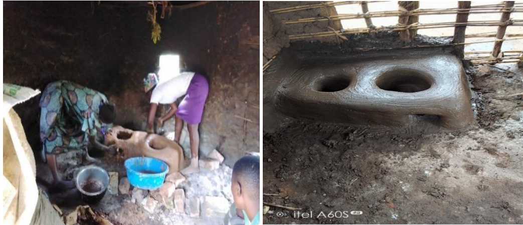
Figure 20: On the left constructing and on right is the new constructed Lorena stove
